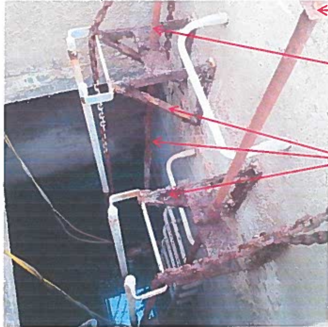
Photo ID: IMG_2016114 - 131559: Dosing Chamber – Effluent pump bracket and operator valve stem corrosion.
