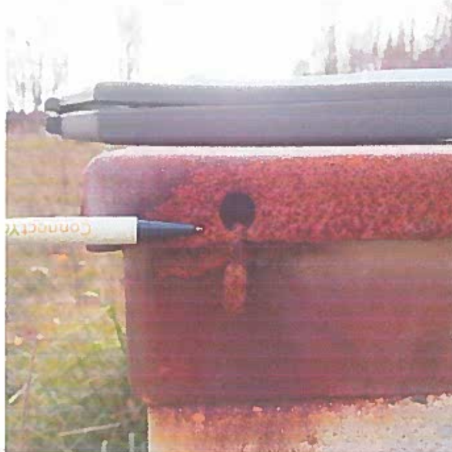
Photo ID IMG_20161114 - 132202: Corrosion of safety chain attachment point on the dosing lid.
